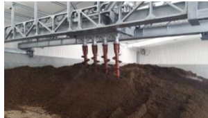
The process of compost production at the East Composting Centre in Kumamoto City.
