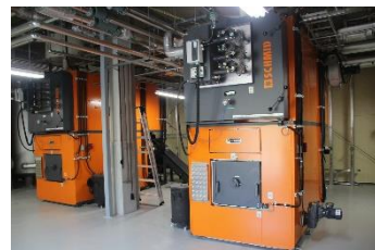
Woody biomass boiler
