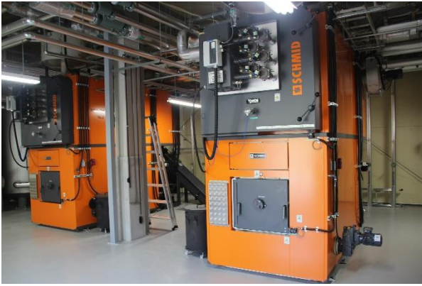
Woody biomass boiler
